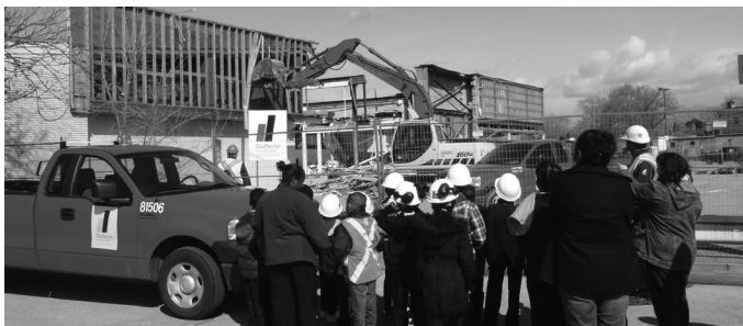
20 children from Royal Day Care visit the construction site next door to learn more about the building demolition and the GTS Project.
