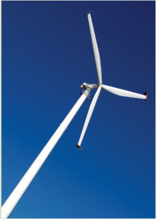
GO propels towards a green future with the introduction of our first wind turbine, at the Lisgar GO Station in Mississauga.
